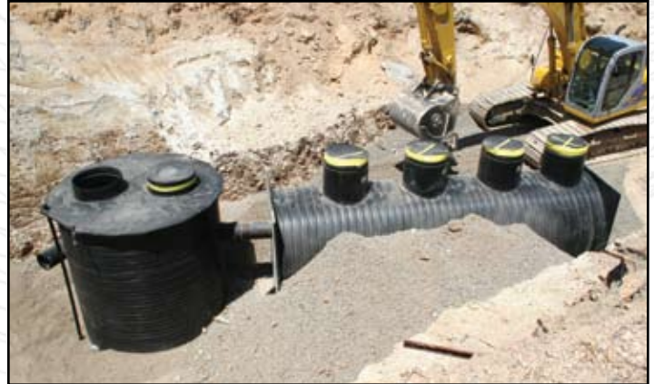
The Aqua-Filter TM Stormwater Filtration System.
