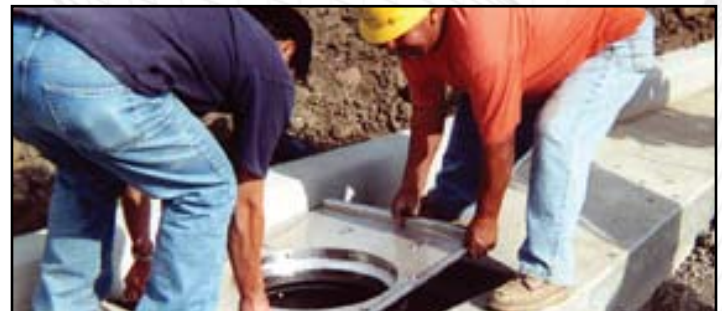
Aqua-Guardian TM system installation in California.
