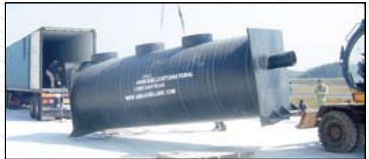
Aqua-Filter TM system installation at an airport in South Korea
