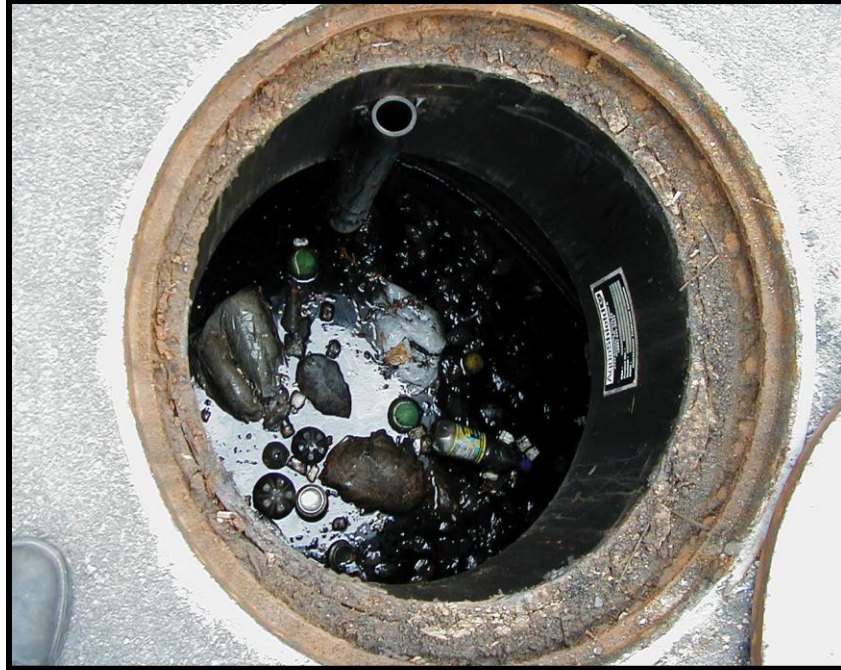
Figure 4. Trash and floatables in an AS-5. Vent pipe is at the top of the photograph.
