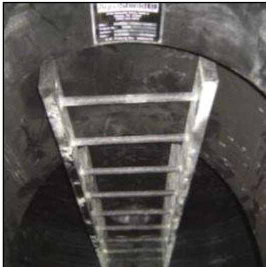
A permanent ingress/egress ladder provides access to filter chamber. Note metal product identification plate above ladder.
