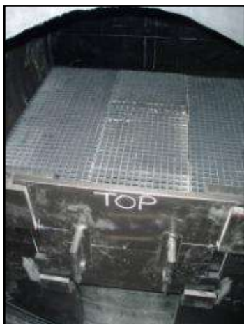
Figure 3. Removable bulkhead door across from ingress/egress ladder at rear of filtration chamber.
