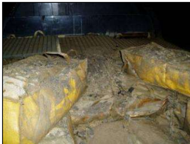
Figure 4. Perlite filter media needs replacement.
